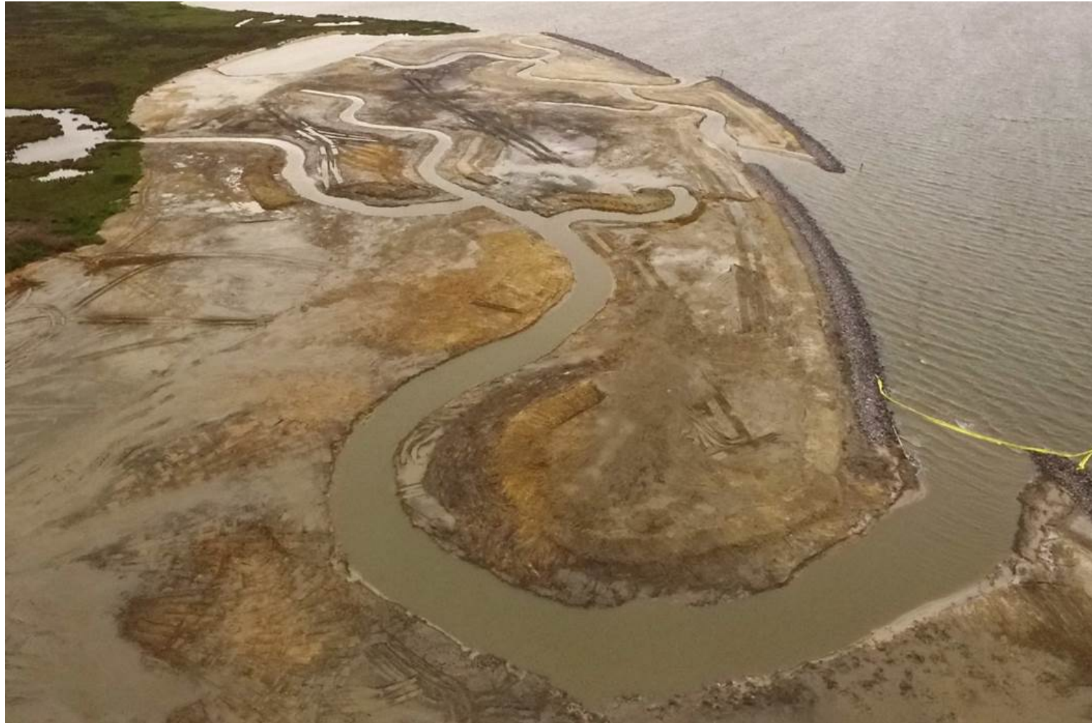
Looking east across Phase 1, East Marsh Creation Area- old meets the new
